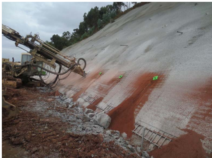
Figure 6. Design of soil nailing based on the occurrence of limestone detected by Electrical Tomography.
