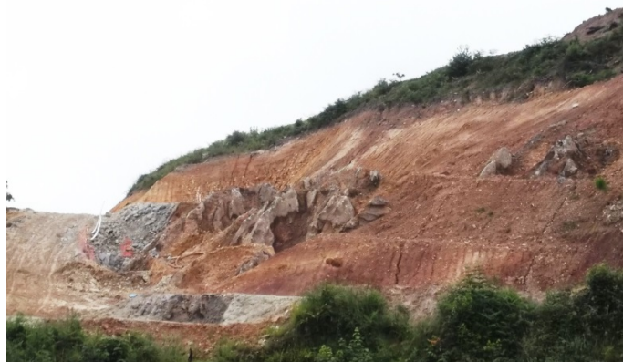
Figure 1. Slope before reinforcement action. Some limestone ridges are visible outcropping at the bottom of the slope.
